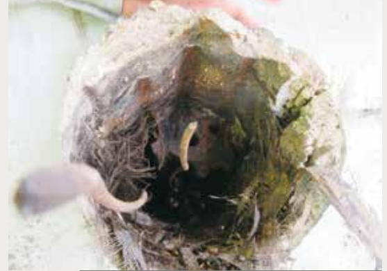
Ruptured cable at the anchorage
